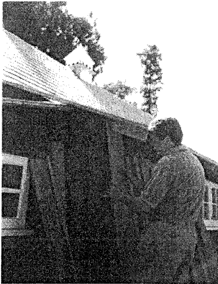
Careful Assembly: General Contractor Bill Abel fits an original plank to the exterior of Walt's Barn.
